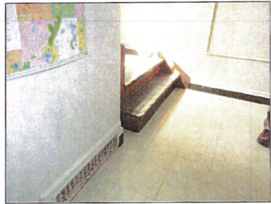
30. Stairs as only access to basement level.
