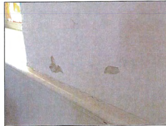
18. Typical of paint peeling from plaster surface
