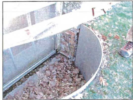
12. Rotted wood window. West elevation of church.
