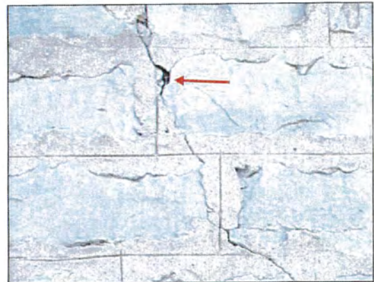
10. Step cracking in mortar at west elevation.
