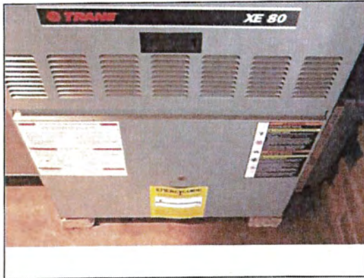
27. TRANE gas fired furnaces (2).
