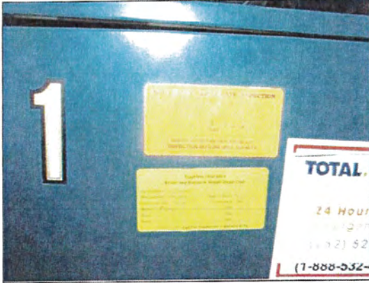
25. Boiler #1 inspection date.
