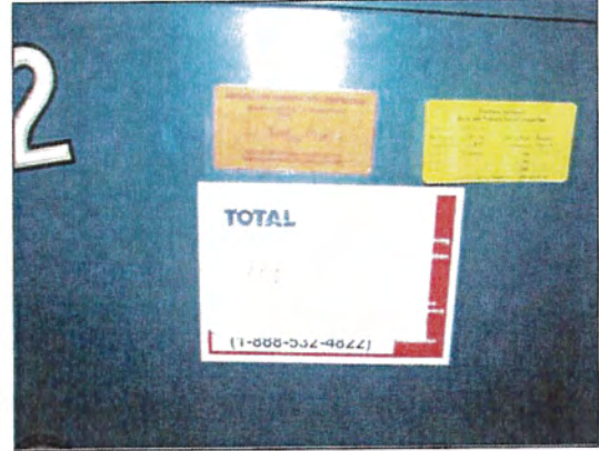
26. Boiler #2 inspection date.
