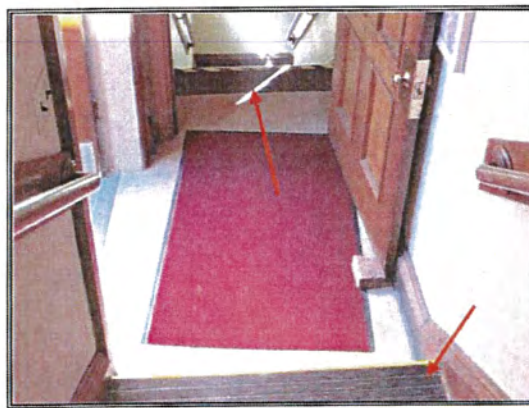
35. Annex entry is below floor line of church (foreground) with stairs leading to basement.
