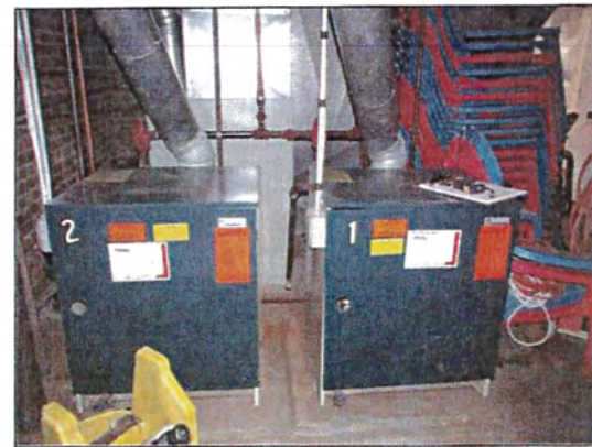
24. Mechanical room, twin Vaillant boilers.
