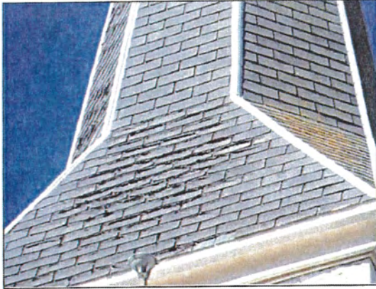
13. Shingle deterioration on steeple, east elevation.
