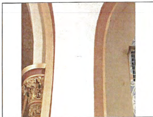
17. Typical of cracks in plaster.
