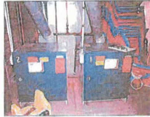
24. Mechanical room, twin Vaillant boilers.
