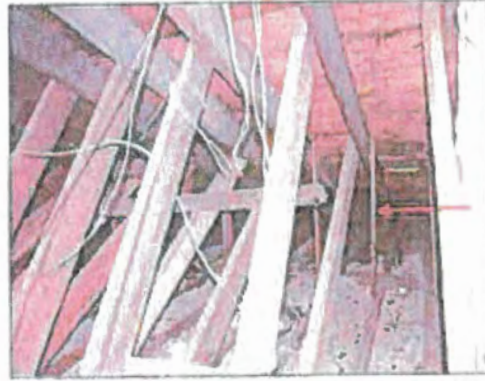
20. View into attic perimeter. Note vertical plaster supports.
