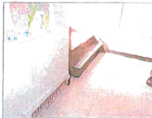
30. Stairs as only access to basement level.
