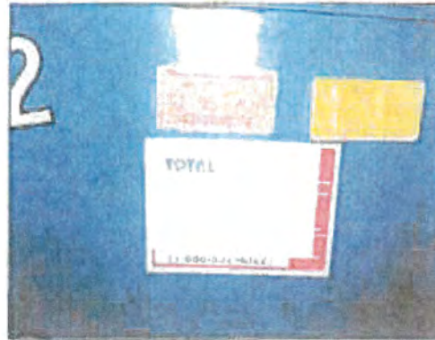
26. Boiler #2 inspection date
