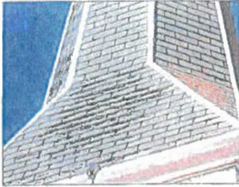
13. Shingle deterioration on steeple, east elevation.
