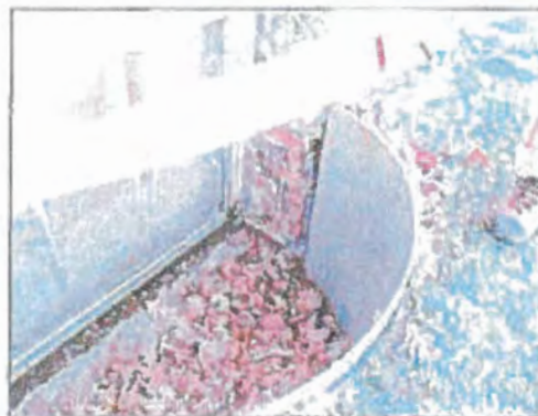
12. Rotted wood window West elevation of church.
