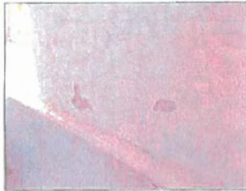
18. Typical of paint peeling from plaster surface
