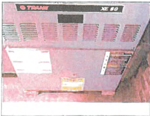
27. TRANE gas fired furnaces (2)
