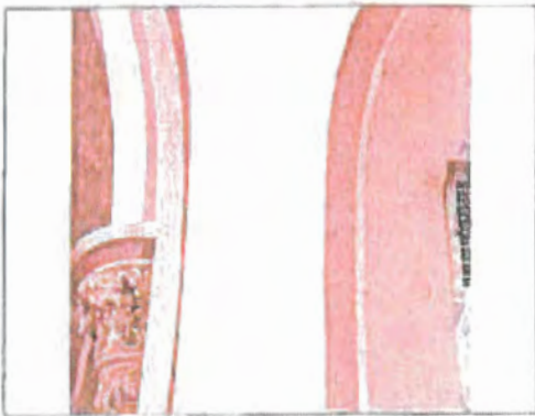
17. Typical of cracks in plaster.
