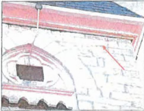
9. Steeple mortar deficiencies
