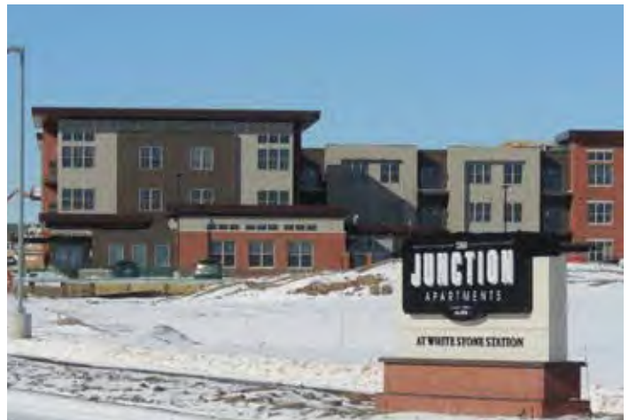
318 apartment units are being constructed at the nearby White Stone Station redevelopment site
