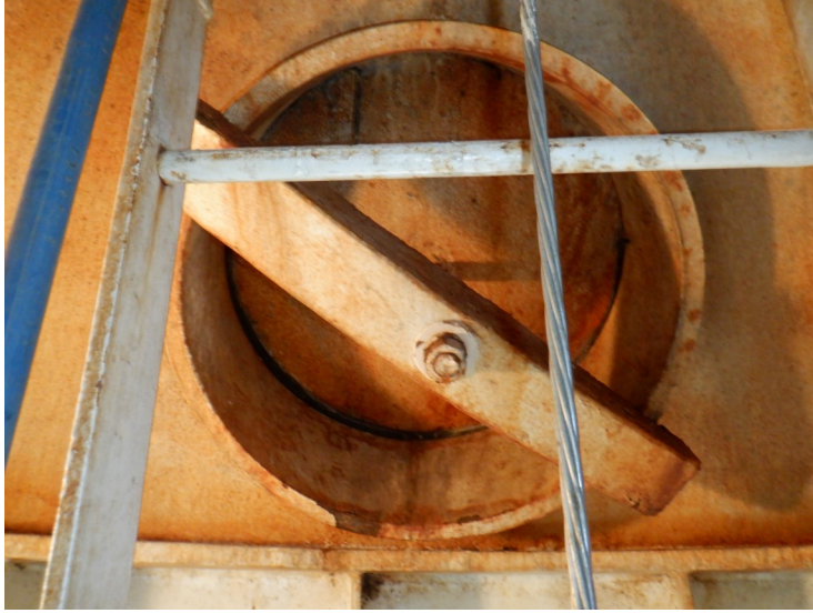
46) Coating failures on the wet interior manway. The manway is in the transition cone.
