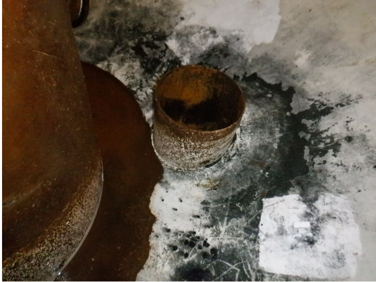
64) There are no deflector bars over the fill/draw pipe in the wet interior.
