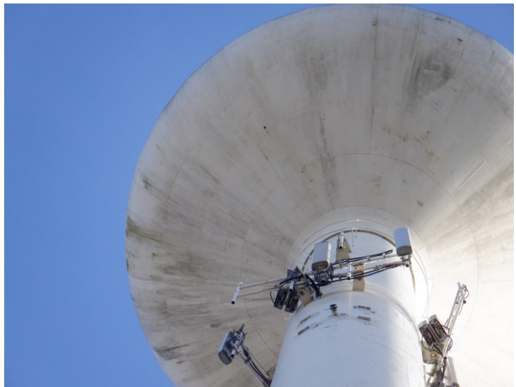
14) A few coating failures on the bowl.
