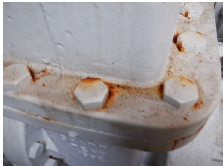
65) There are spot coating failures on the bolts and flanges.
