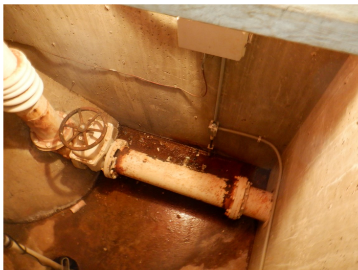
66) Coating failures on the pit piping.
