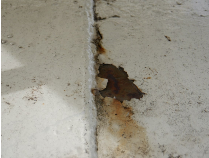
22) Spot coating failures on the roof.
