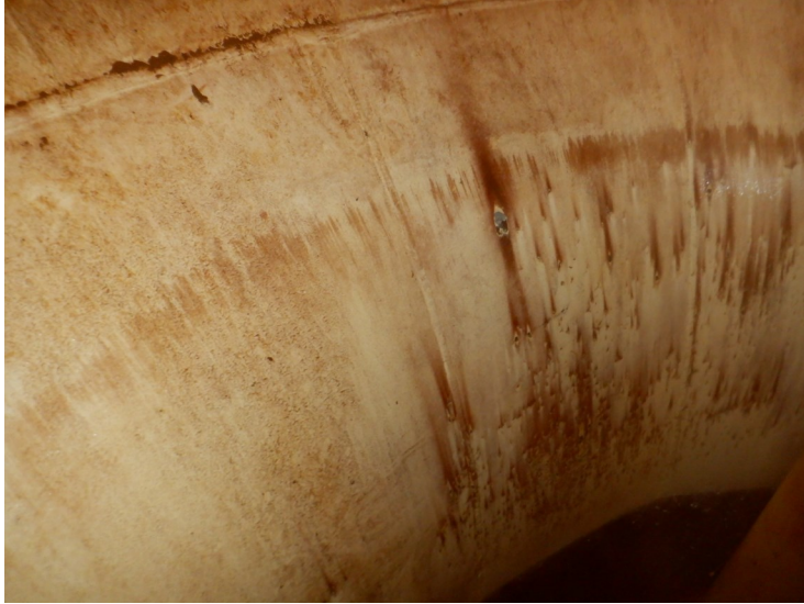
61) Coating failures in the transition cone.
