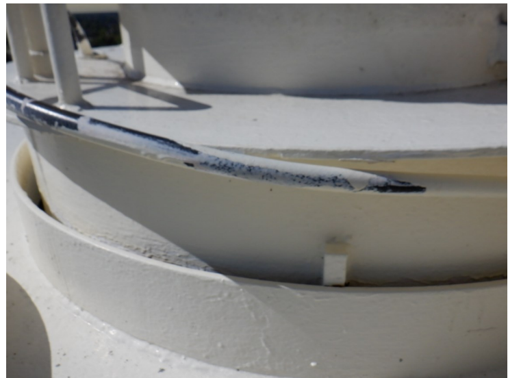
20) There is no cover over the access tube air gap.
