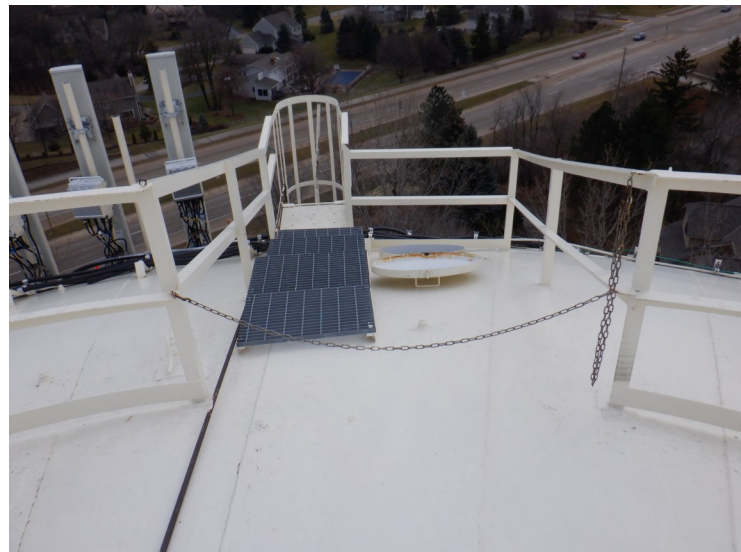
26) The step-off platform and roof hatch are surrounded by a handrail that is in good condition.
