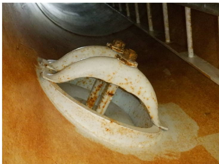
48) Coating failures on the wet interior manway.
