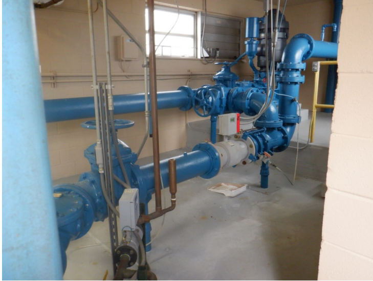
19) Coating on the piping in the pumphouse is in good condition overall.
