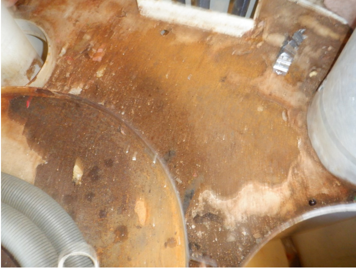
43) Coating failure on the top platform.
