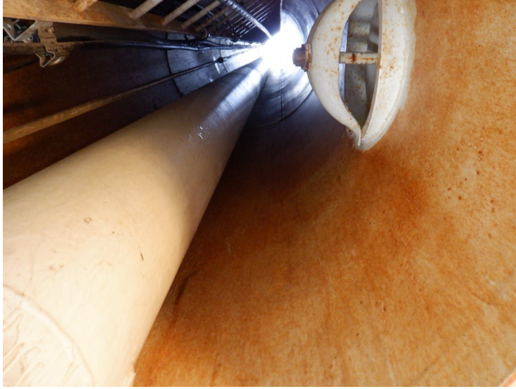
46) Extensive rust bleedthrough in the access tube.
