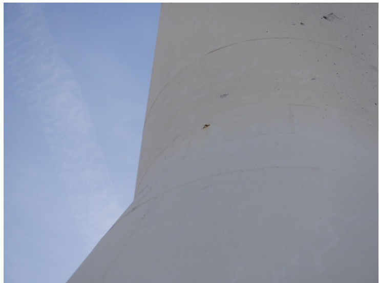
11) Coating failures on the riser.
