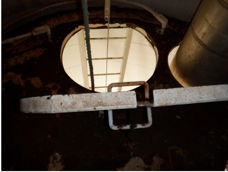
34) The ladder opening in the condensate platform is equipped with a hinged cover.
