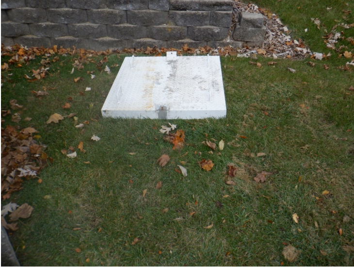
7) The roof hatch covers are in good condition with some coating erosion.
