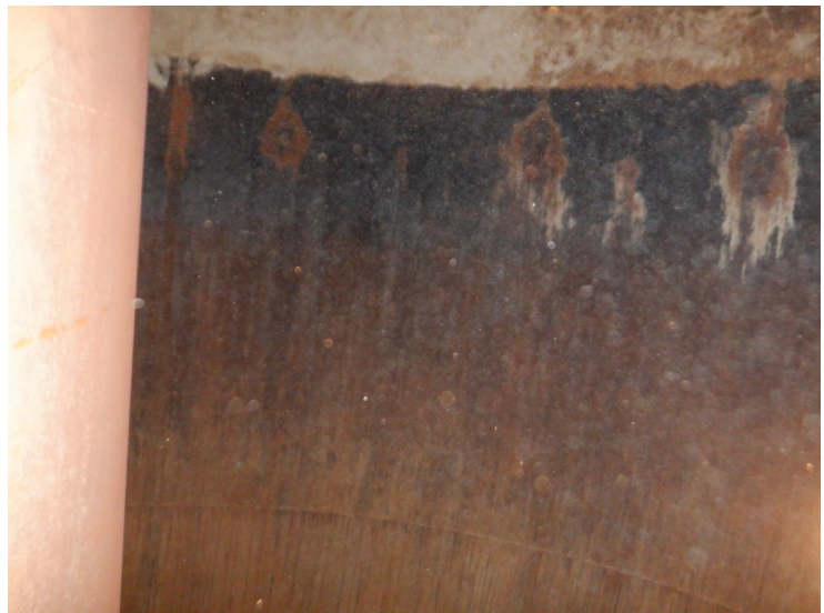
53) There is heavy mineral staining on the wet interior sidewall but no coating failures.
