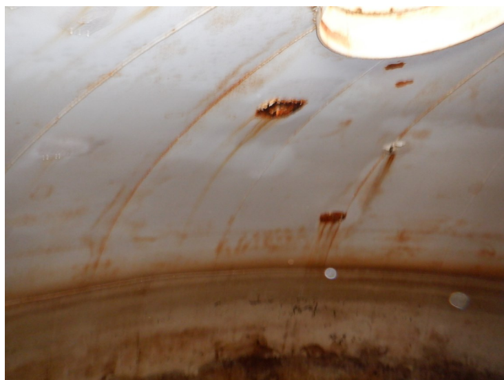
51) Coating failures on the wet interior roof.
