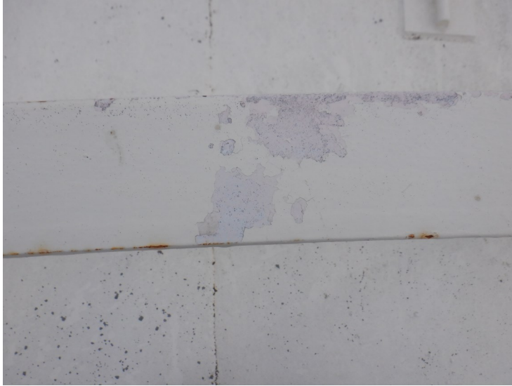
28) There is delamination along the handrail.
