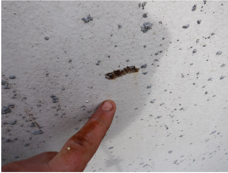
16) There are several small spot coating failures on the sidewall.
