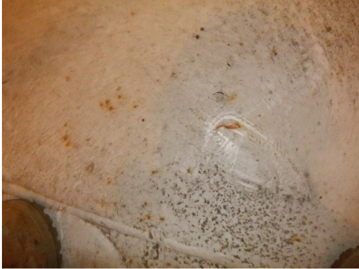
31) Minor coating failures on the condensate platform.
