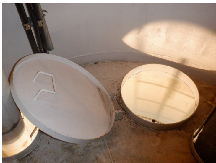
30) The ladder opening at the condensate platform is equipped with a hinged cover.
