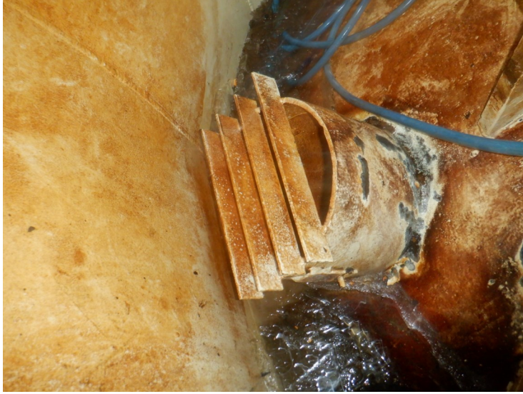
64) There are deflector bars over the fill/draw pipe in the wet interior.
