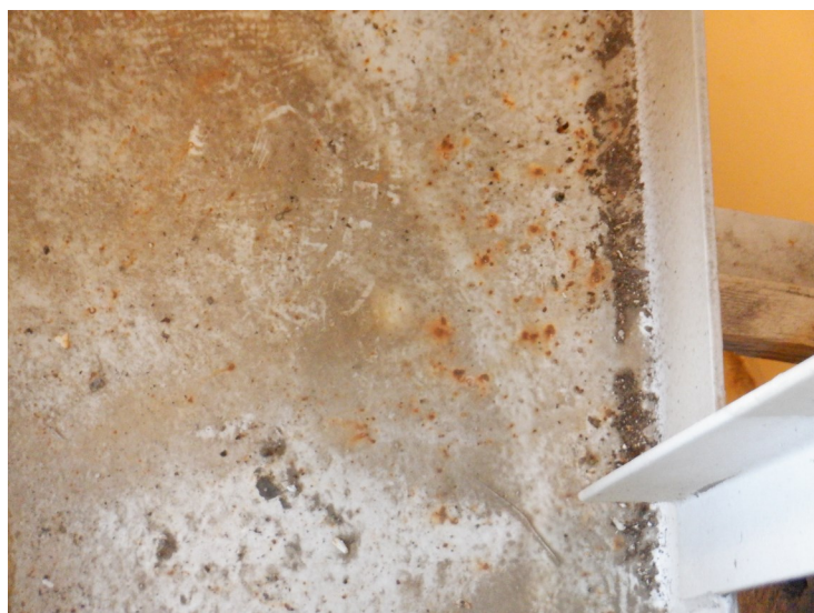
39) Minor coating failures on the top platform.
