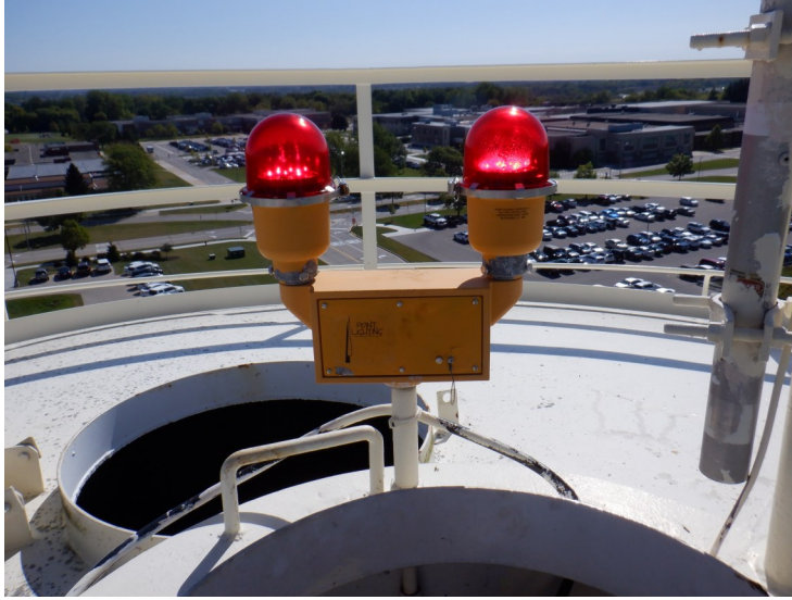
25) The double aviation light was operating properly during the inspection.
