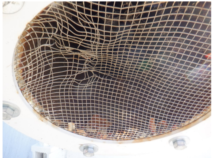
5) The screen at the overflow discharge is intact but deformed and oversized.
