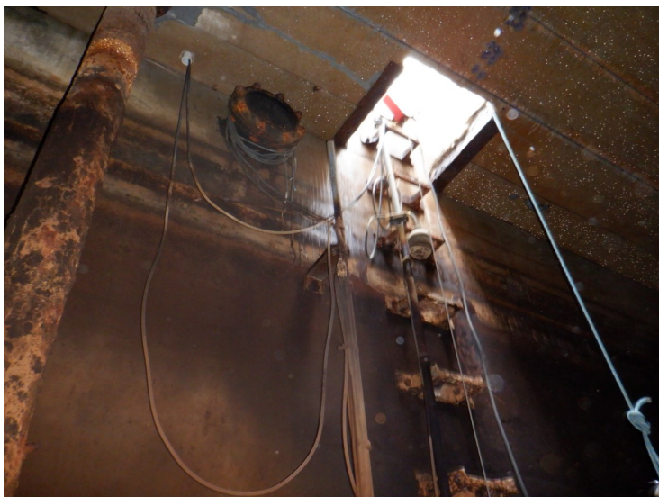
15) The metal wet interior appurtenances are not coated.
