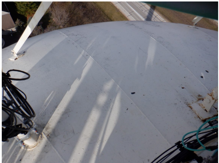
20) Coating failures on the roof.
