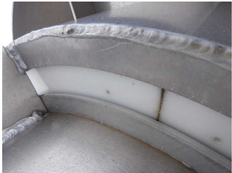
35) The pressure plate is in good condition.
