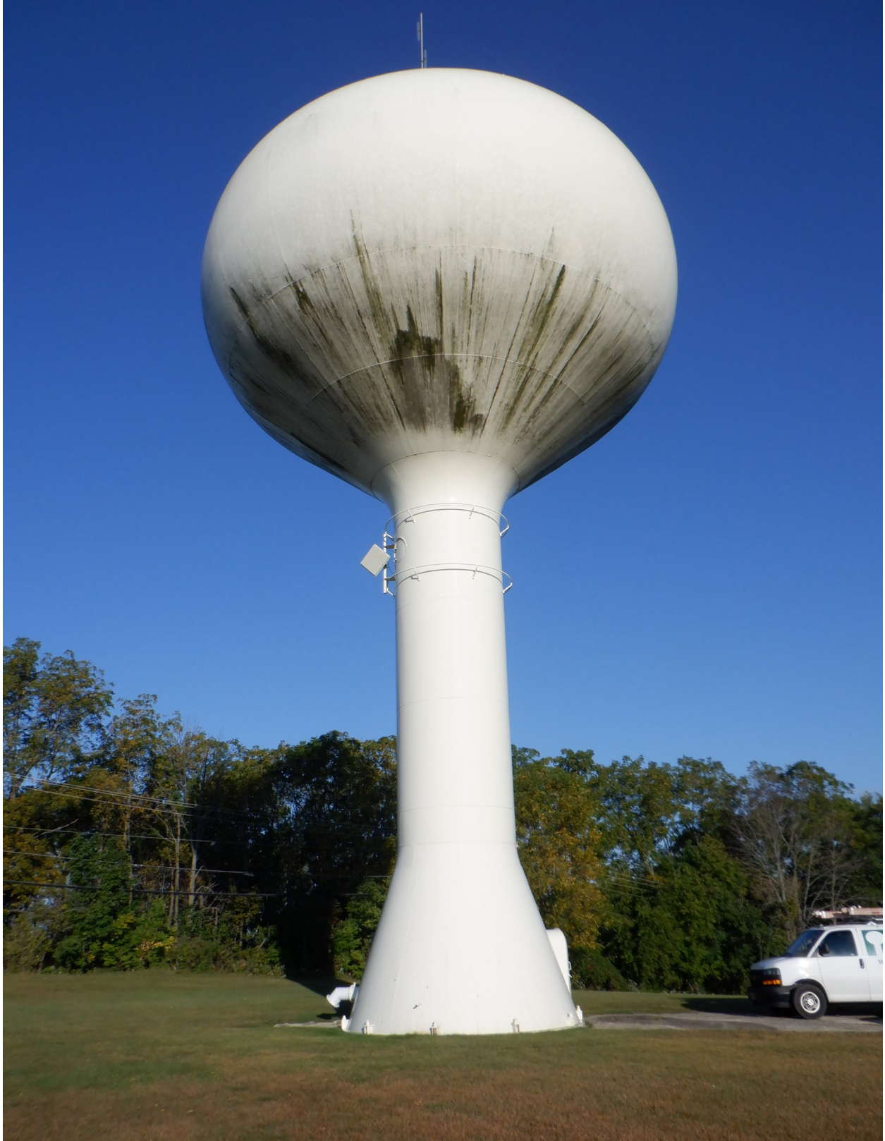
250,000 gallon spheroid (Lake Street) elevated water storage tank owned by the Village of Pewaukee, Wisconsin.
