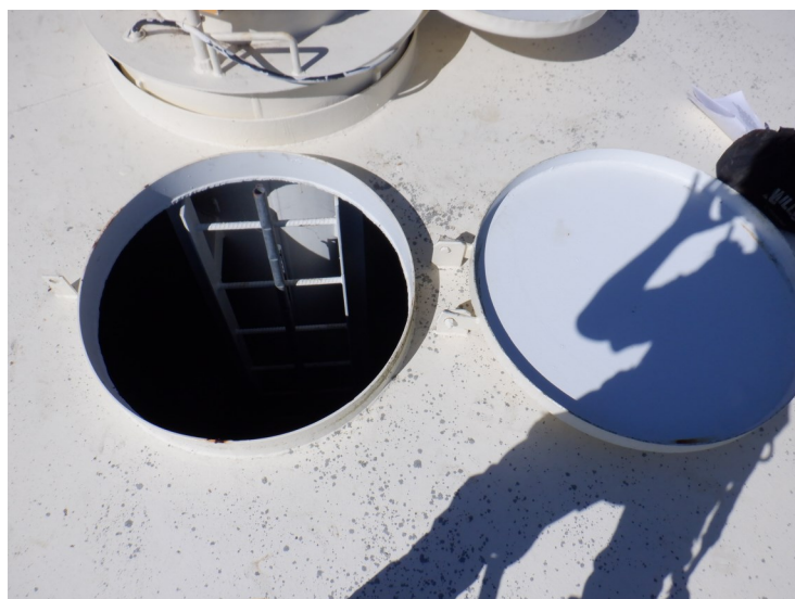
18) The wet interior roof hatch is in good condition. A gasket was installed on the hatch during the inspection.
