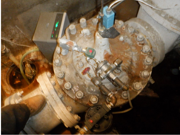
67) Minor coating failures on the pit piping.
