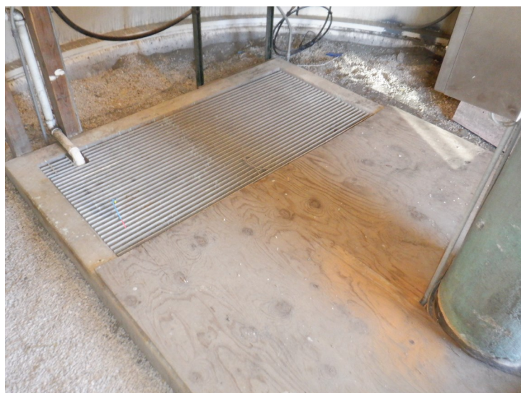
66) The cover over the pit in the basebell is in good condition.
