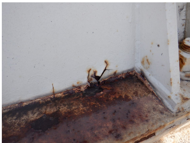
6) Coating failures on the baseplate.
