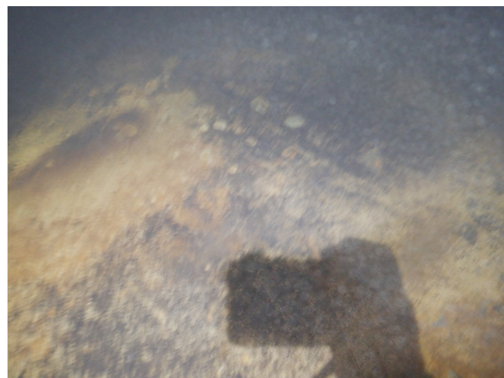
18) There is some erosion of the elastomeric coating on the floor.
