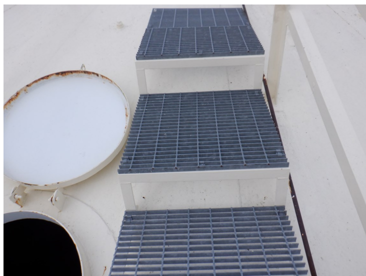
24) The steps to the center of the roof are in good condition.
