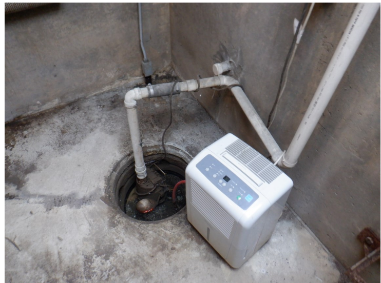
62) There is a sump pump in the pit.
