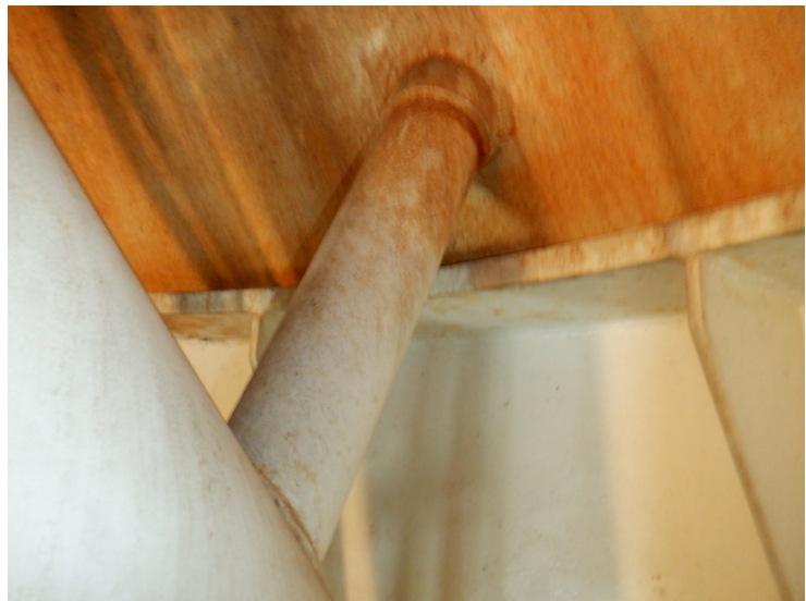
47) There is a drain pipe routed to the overflow pipe.
