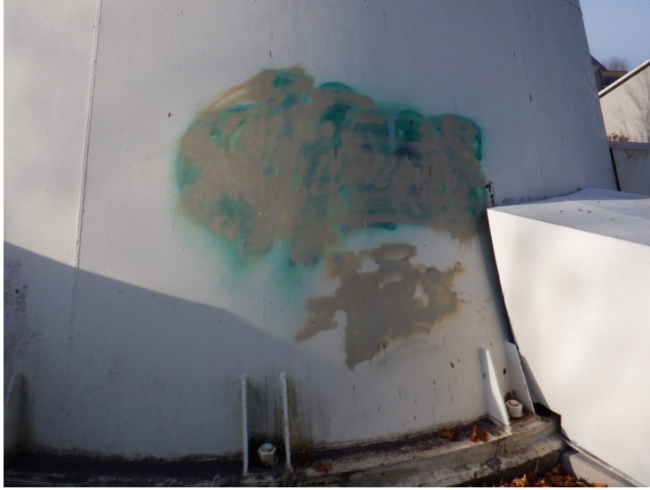
7) Coating failures on the basebell.
