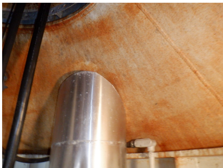
45) Rust bleedthrough on the transition cone.
