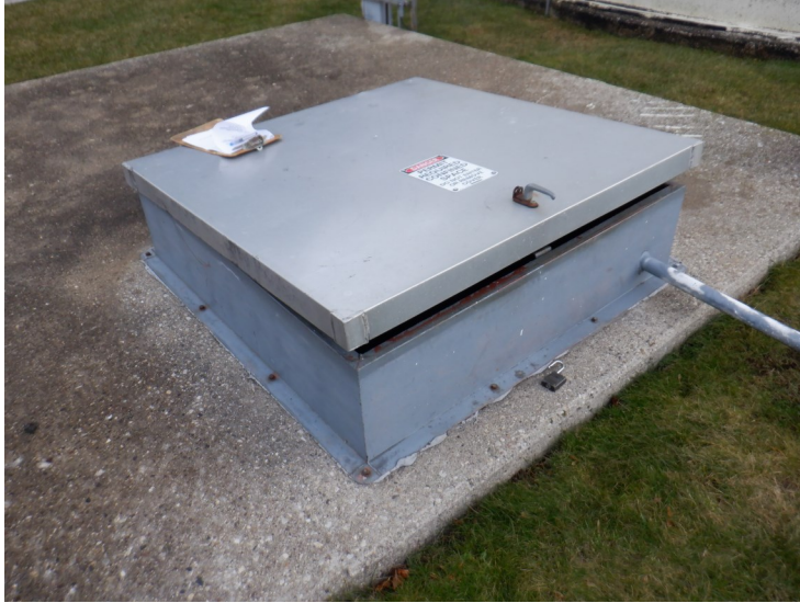
61) There is a pit adjacent to the tank. The pit has a metal hatch that is in good condition.
