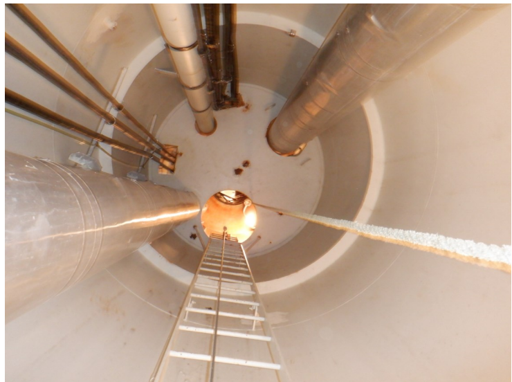
41) The riser ladder is in good condition. The ladder is equipped with a fall prevention device.
