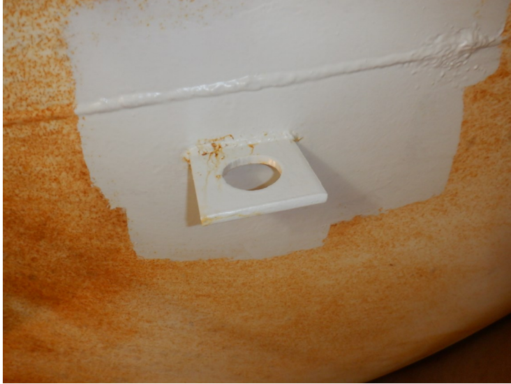
43) There is a rigging lug on the bowl above the top platform hatch.
