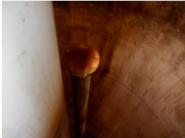
56) There is an abandoned pipe with a blind flange in the wet interior that extends up near the high-water level.
