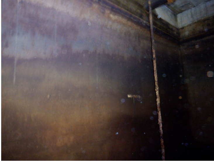
13) Elastomeric coating failures on the wet interior sidewall.
