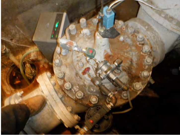
67) Minor coating failures on the pit piping.
