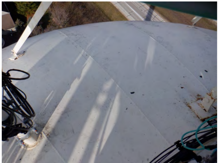
20) Coating failures on the roof.
