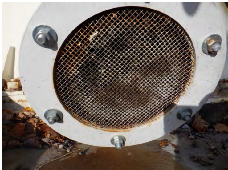
5) The screen at the overflow pipe discharge is intact with no gaps.
