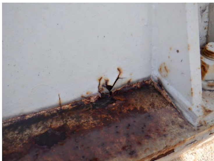
6) Coating failures on the baseplate.
