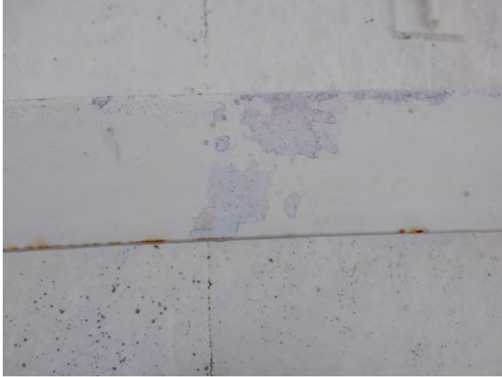
28) There is delamination along the handrail.
