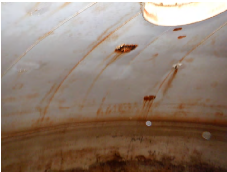
51) Coating failures on the wet interior roof.
