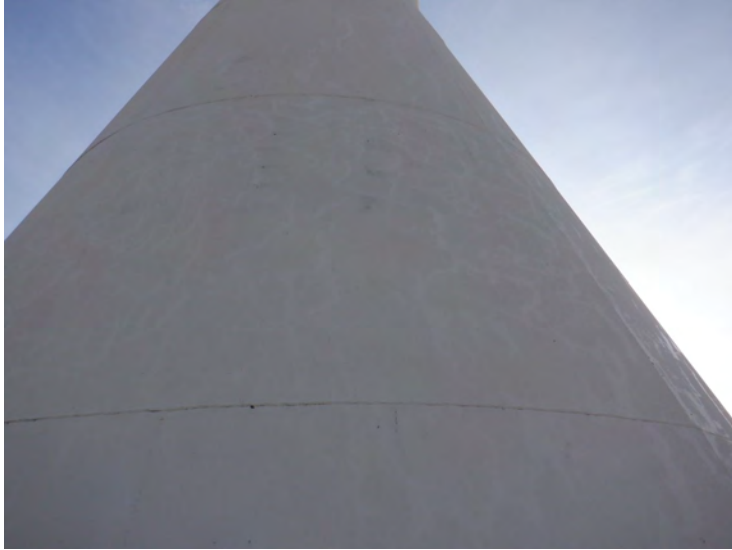
10) The basebell coating is in fair condition overall.
