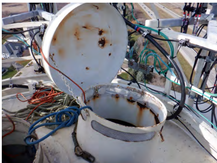
24) There is not a gasket on the wet interior roof hatch.
