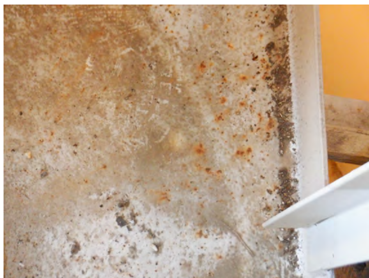
39) Minor coating failures on the top platform.
