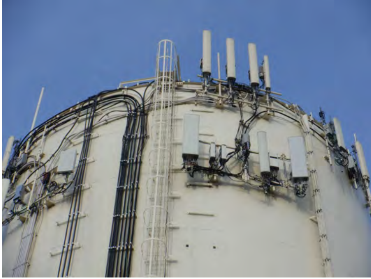
19) There are antennas mounted at the top of the sidewall.
