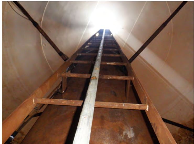
59) The wet interior ladder is in good condition. The ladder is equipped with a fall prevention device.
