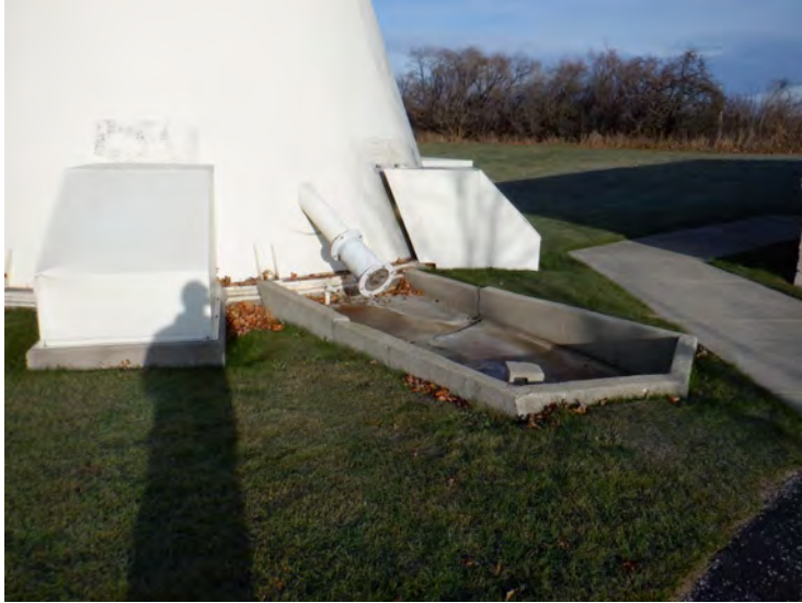
4) The overflow pipe discharges to a splash pad.
