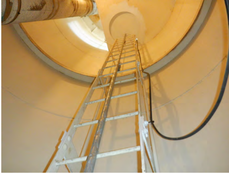
37) The riser ladder is in good condition. The ladder is equipped with a fall prevention device.
