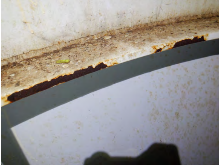
37) Coating failure on a stiffener in the dry riser.
