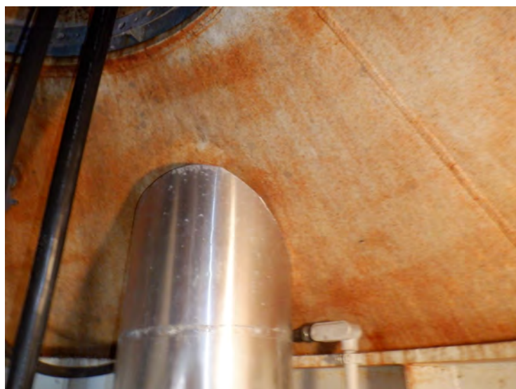
45) Rust bleedthrough on the transition cone.
