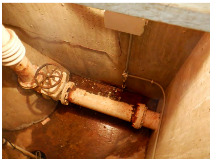
66) Coating failures on the pit piping.
