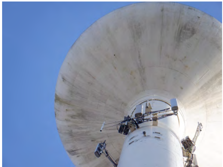
14) A few coating failures on the bowl.
