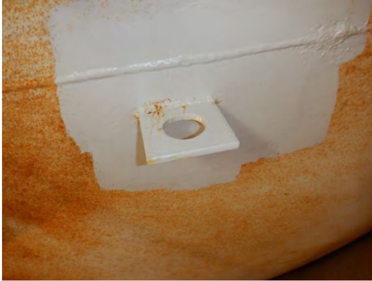
43) There is a rigging lug on the bowl above the top platform hatch.
