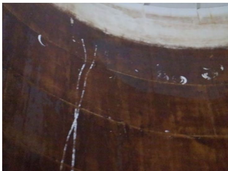
48) There are scratches in the mineral staining near the high-water level.
