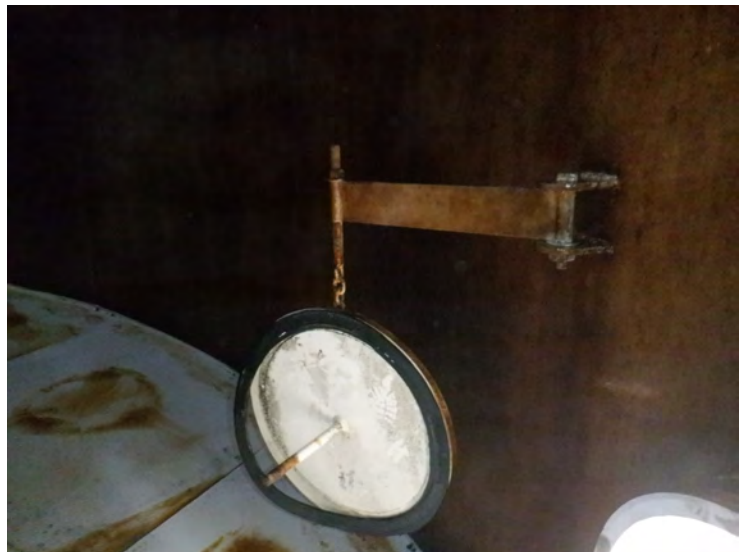
53) The manway covers are held by a davit arm that is in good condition.
