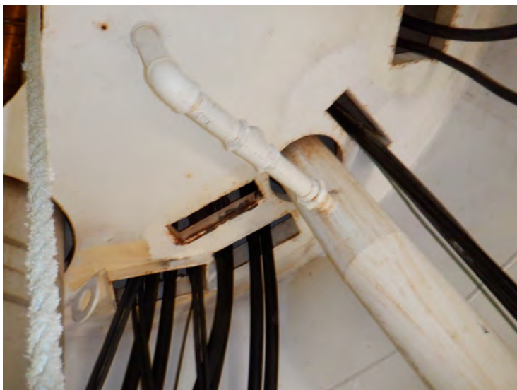
33) There is a check valve on the condensate platform drain.
