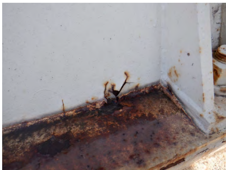
6) Coating failures on the baseplate.
