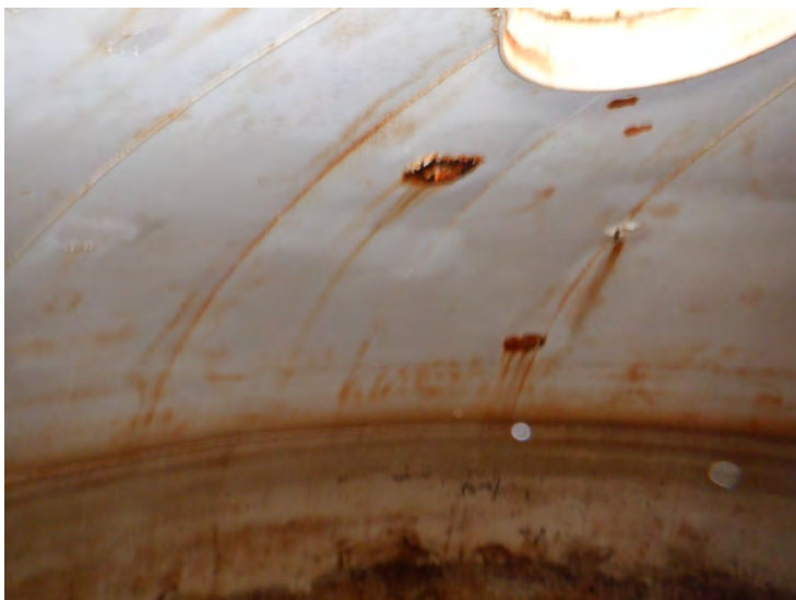
51) Coating failures on the wet interior roof.
