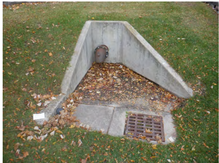
2) The overflow pipe discharges to a catch basin.
