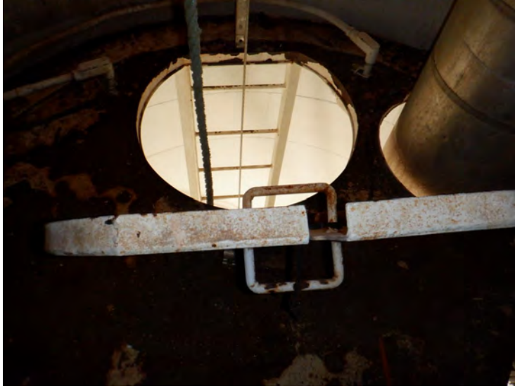
34) The ladder opening in the condensate platform is equipped with a hinged cover.
