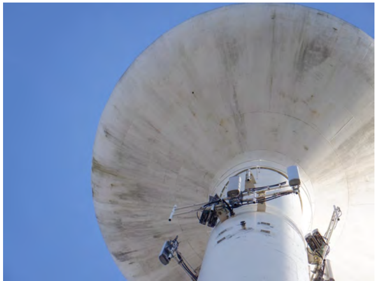
14) A few coating failures on the bowl.
