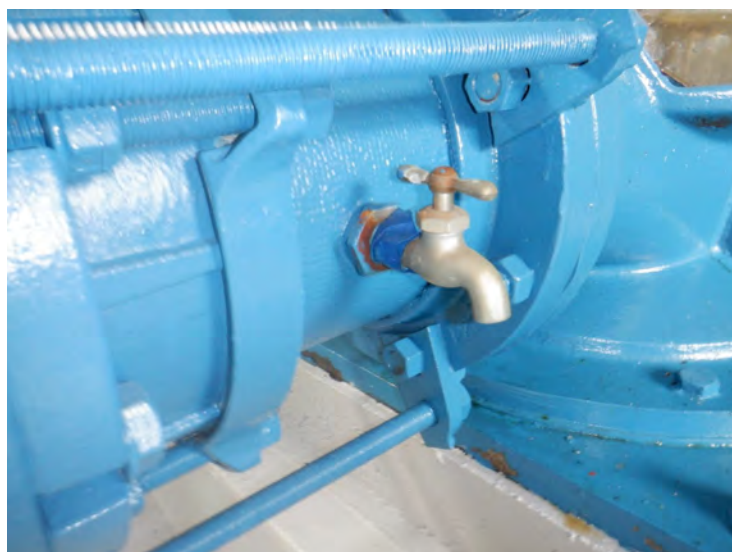
21) The sample tap in the pumphouse is in good condition.
