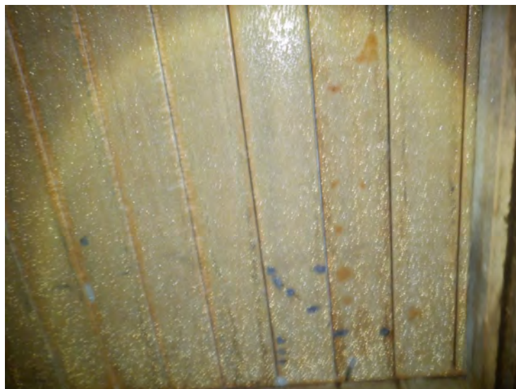
9) Rusting at the surface of the wet interior roof.
