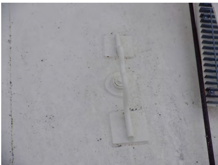
30) Some of the roof rigging couplings have safety clips that are in good condition.
