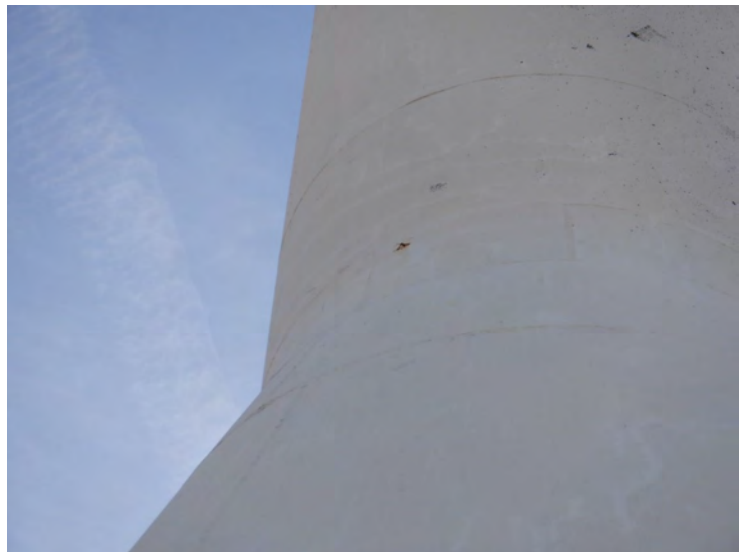
11) Coating failures on the riser.
