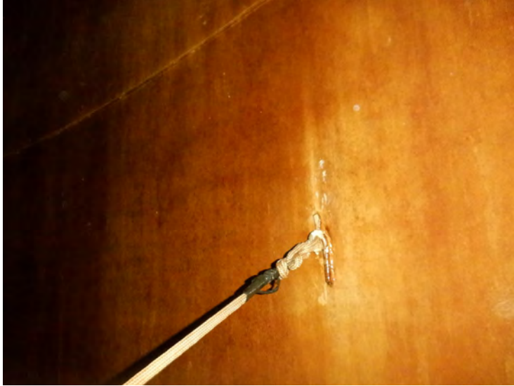
52) There are cathodic protection clips on the sidewall.
