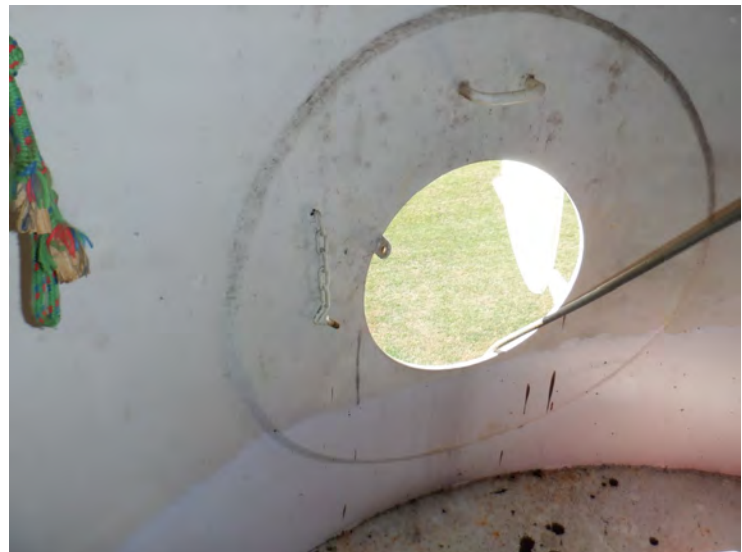
41) There is a handhold above the painter's hatch at the top of the riser.
