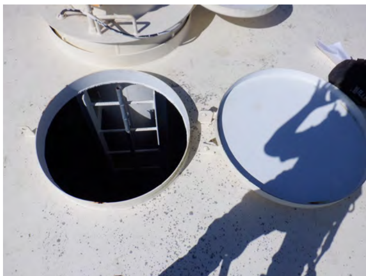
18) The wet interior roof hatch is in good condition. A gasket was installed on the hatch during the inspection.
