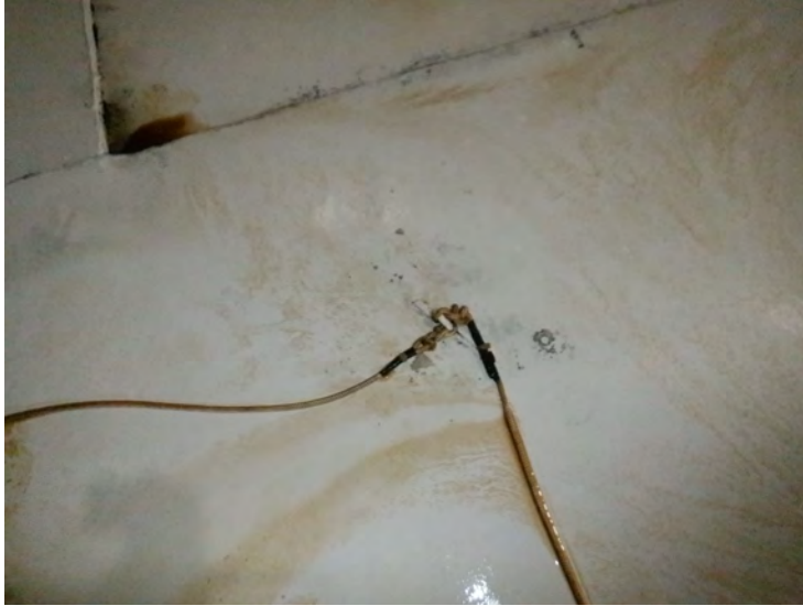
58) There are cathodic clips on the floor.
