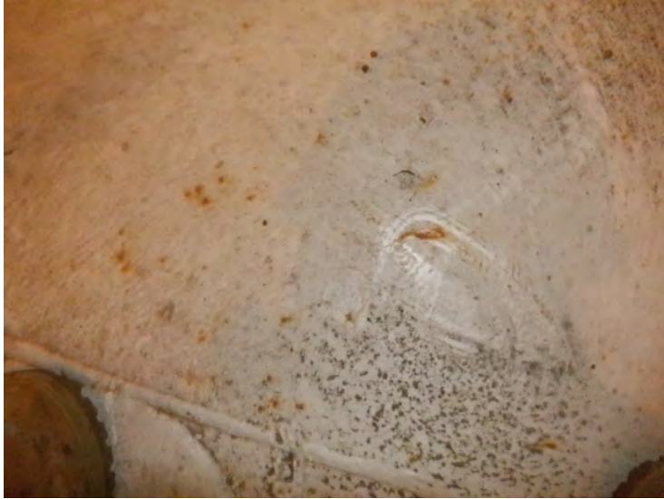
31) Minor coating failures on the condensate platform.
