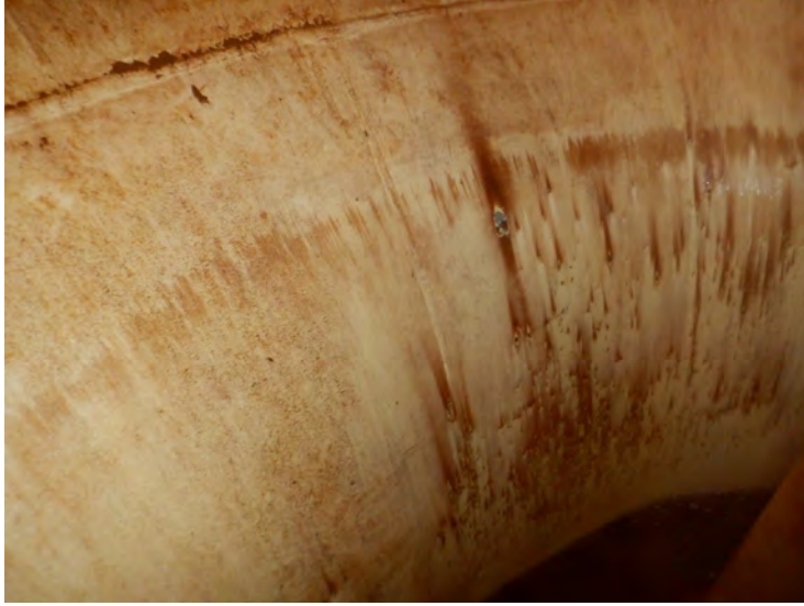
61) Coating failures in the transition cone.
