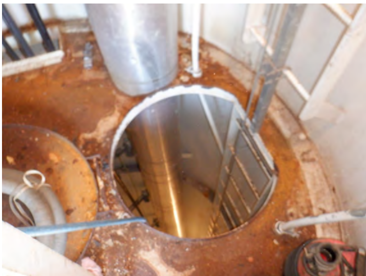
42) The ladder opening at the top platform is equipped with a hinged cover.
