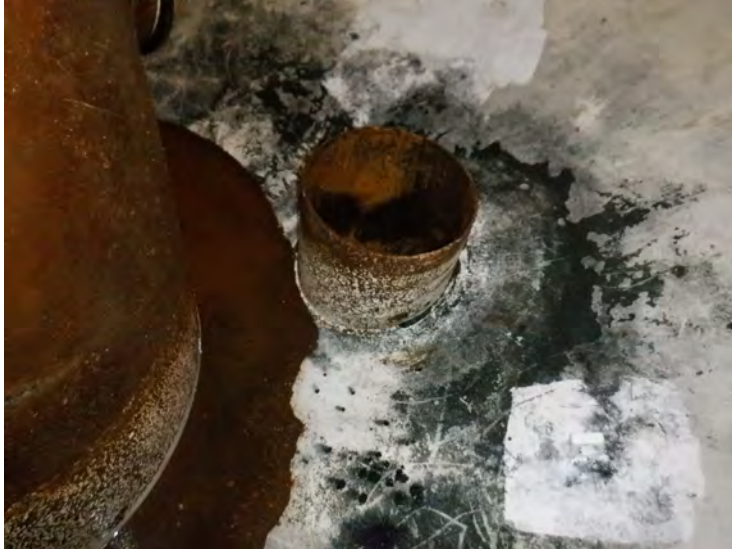
64) There are no deflector bars over the fill/draw pipe in the wet interior.
