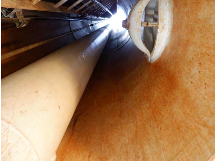
46) Extensive rust bleedthrough in the access tube.
