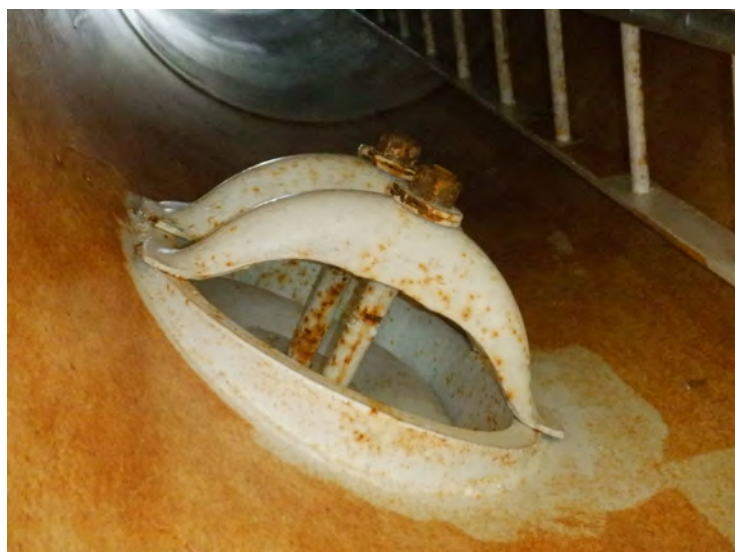
48) Coating failures on the wet interior manway.
