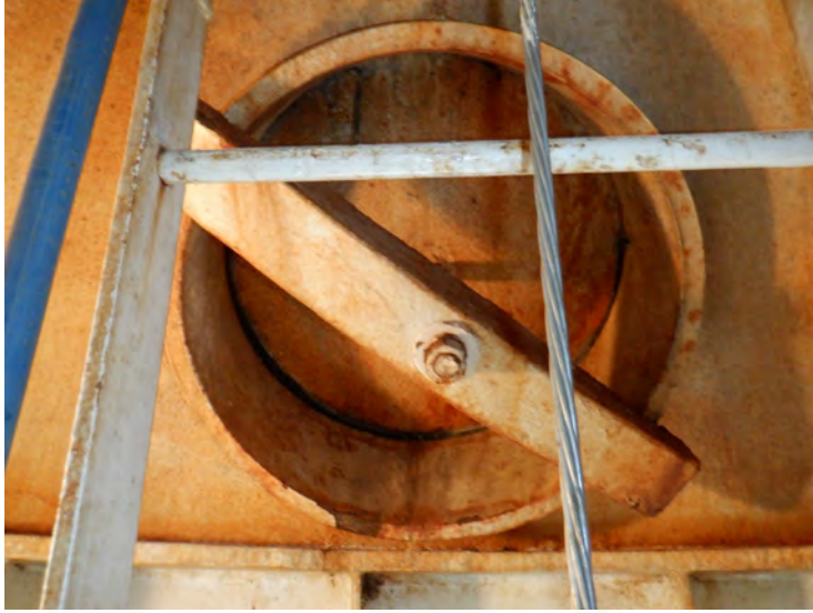
46) Coating failures on the wet interior manway. The manway is in the transition cone.
