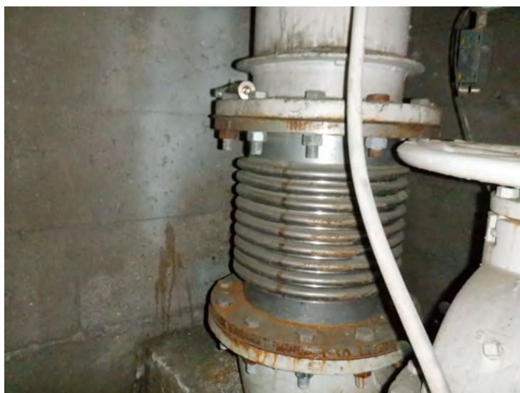
69) The bellows type expansion joint on the fill/draw pipe is in good condition.
