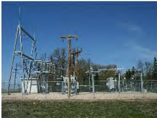
Image: Electrical substation
