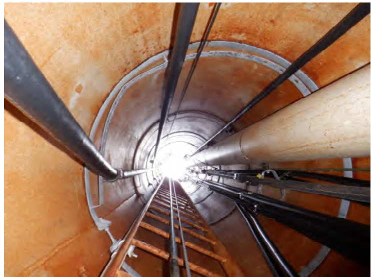
50) The access tube ladder is in good condition. The ladder is equipped with a fall prevention device.
