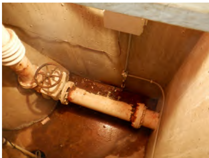
66) Coating failures on the pit piping.
