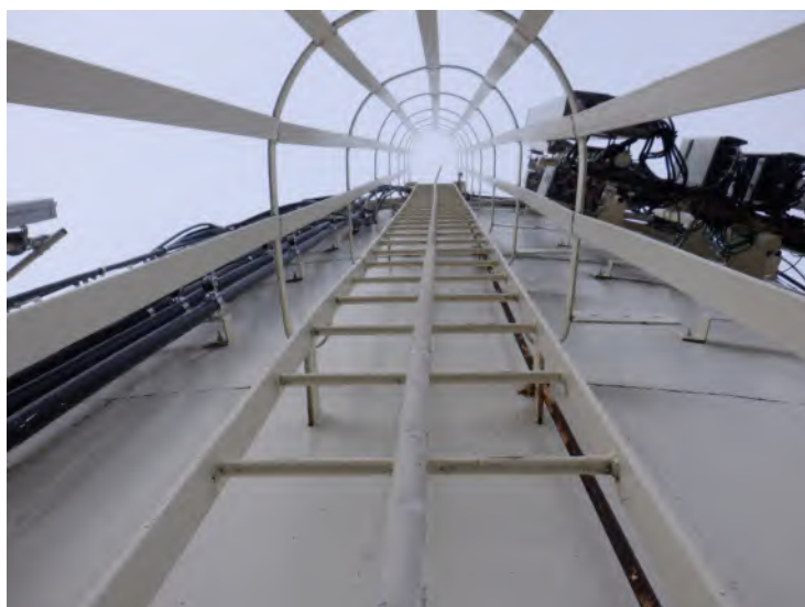
12) The sidewall ladder fall prevention device is coated.
