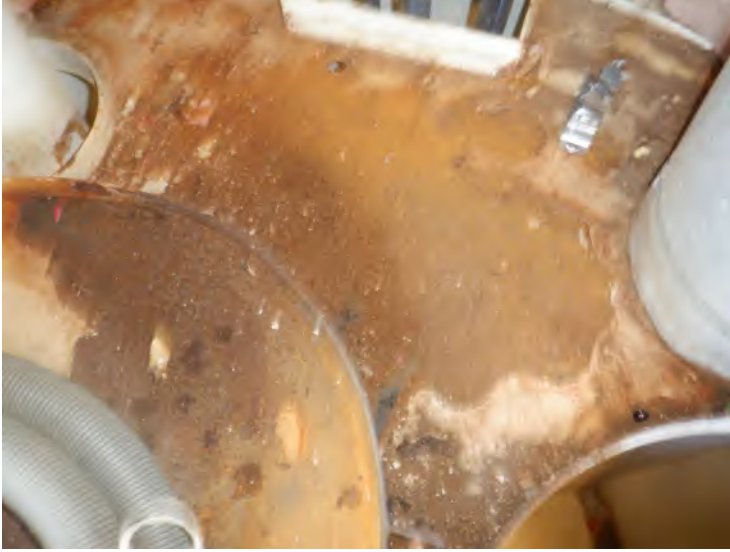
43) Coating failure on the top platform.
