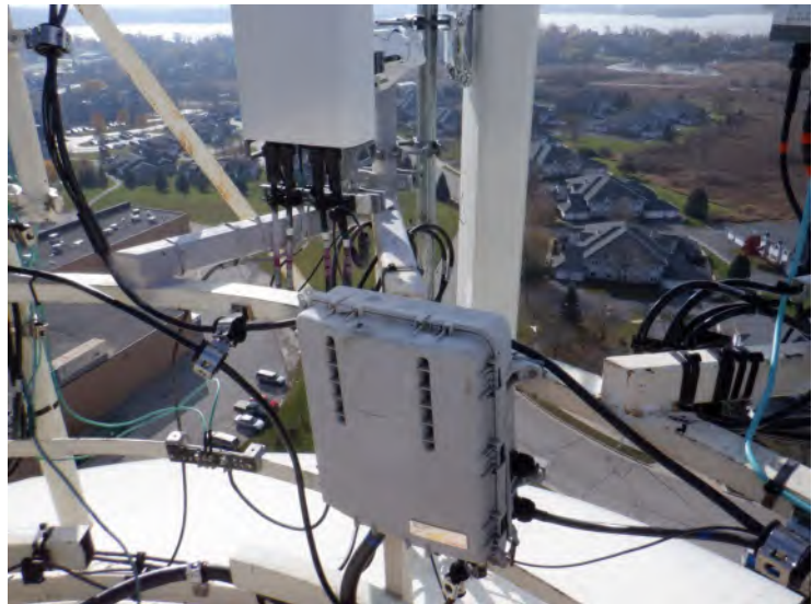
23) The roof handrail is in good condition. There are antennas attached to the roof handrail. There is not a painter's railing on the roof
