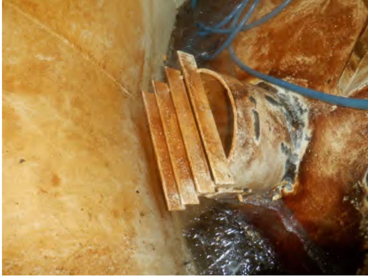
64) There are deflector bars over the fill/draw pipe in the wet interior.
