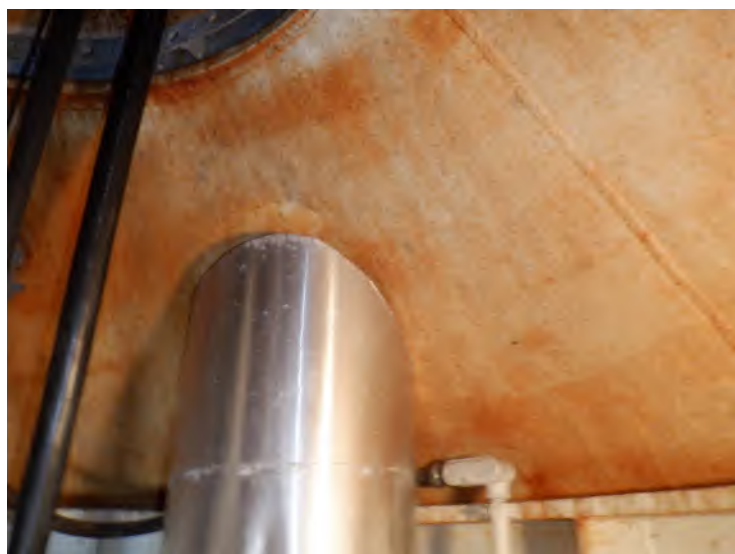
45) Rust bleedthrough on the transition cone.
