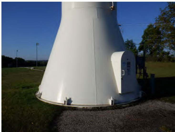
6) There are no coating failures on the basebell.
