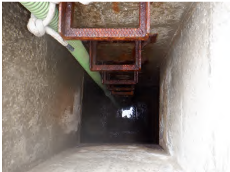
8) The ladder cleats from the roof to the floor are in good condition.
