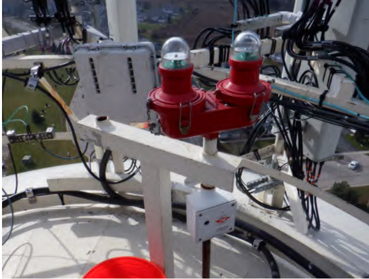
28) The aviation light was operating properly during the inspection.
