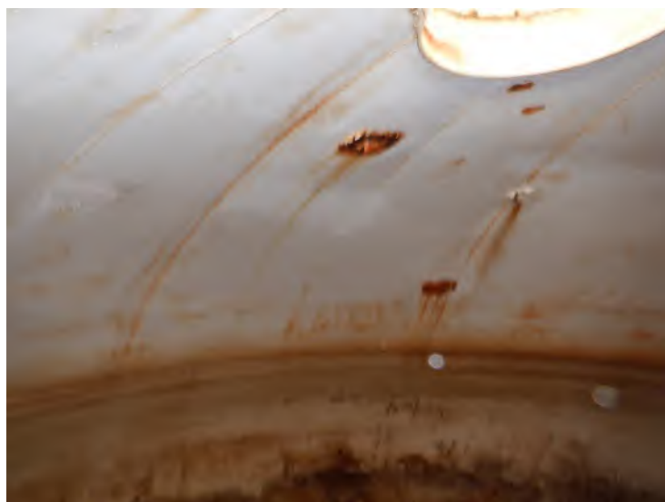
51) Coating failures on the wet interior roof.
