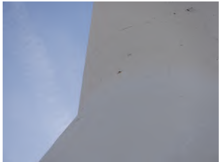
11) Coating failures on the riser.
