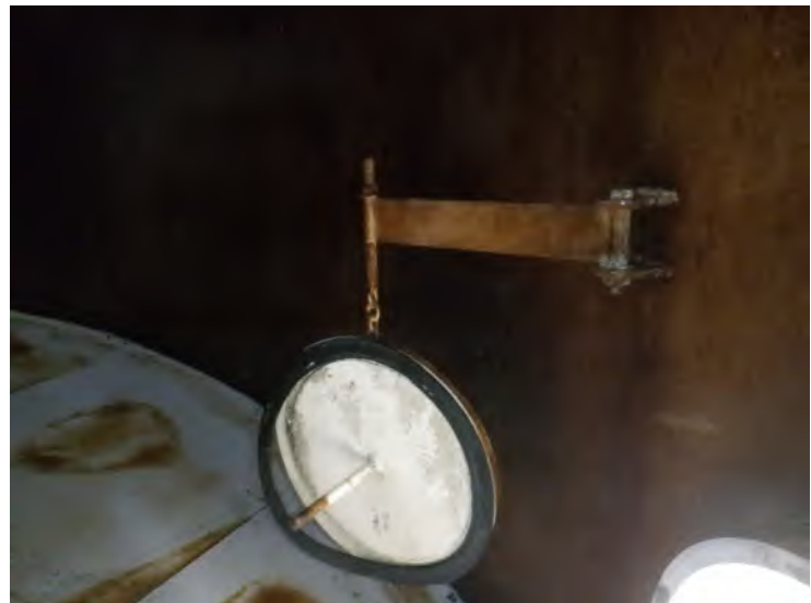
53) The manway covers are held by a davit arm that is in good condition.
