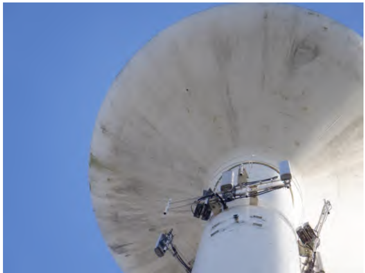
14) A few coating failures on the bowl.
