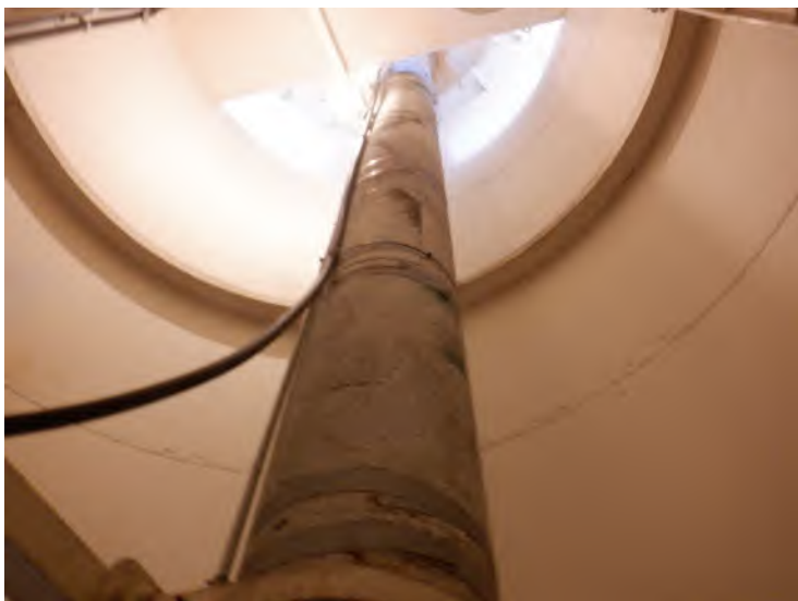
36) There is no cover over the fill/draw pipe insulation.
