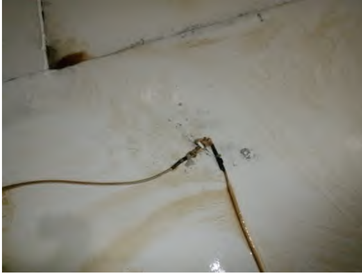
58) There are cathodic clips on the floor.
