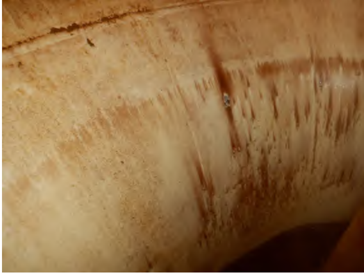
61) Coating failures in the transition cone.
