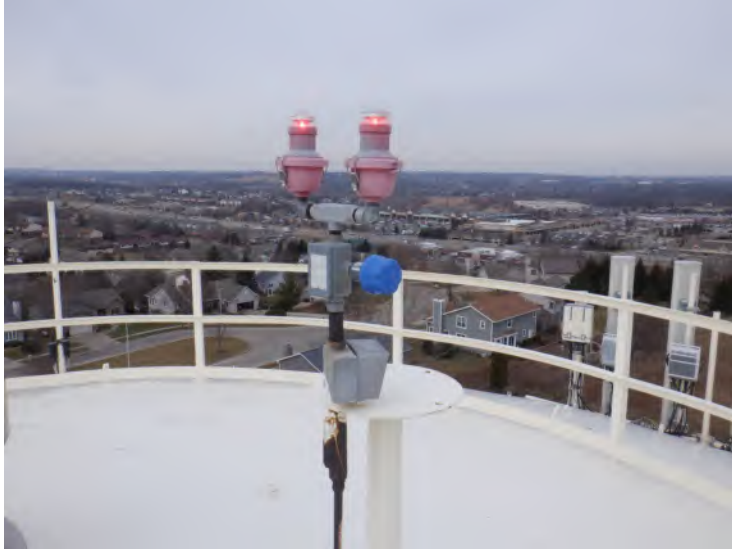
31) The double aviation light is in good condition.
