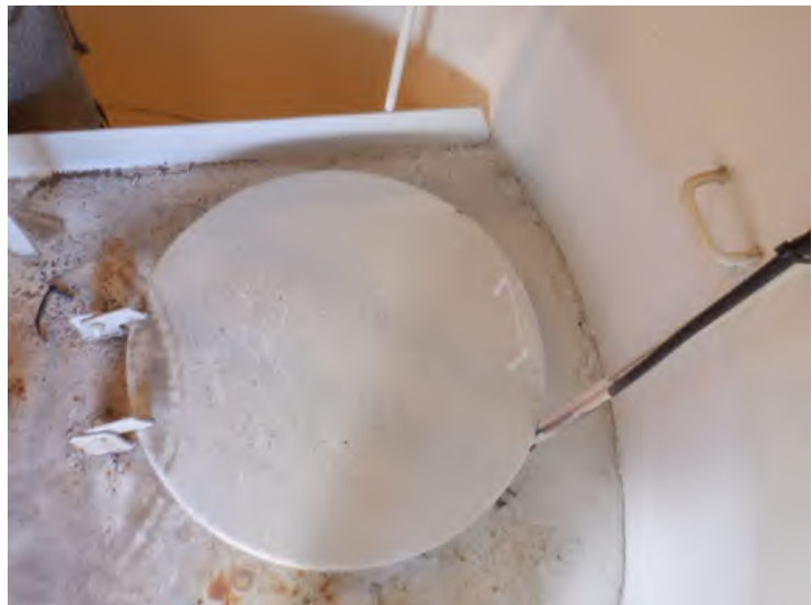
38) The ladder opening at the top platform is equipped with a hinged cover.
