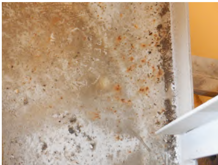
39) Minor coating failures on the top platform.
