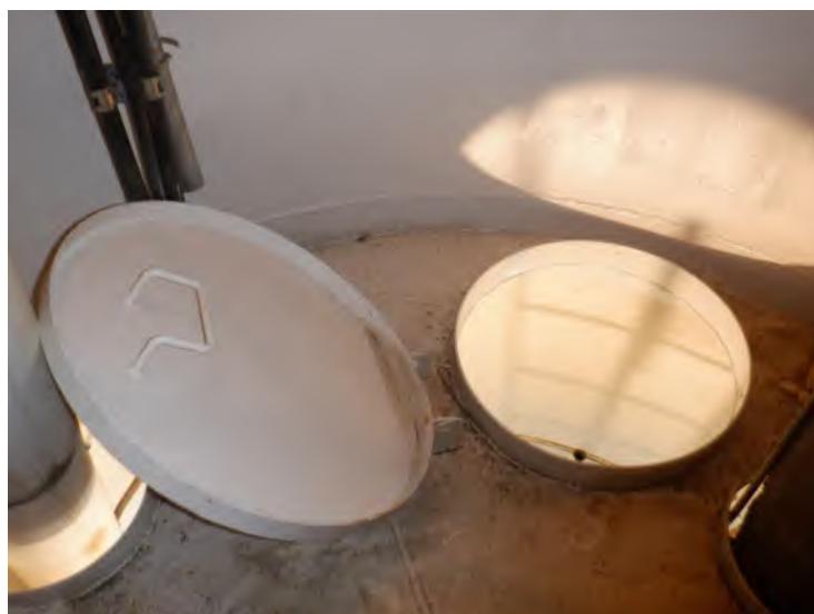
30) The ladder opening at the condensate platform is equipped with a hinged cover.
