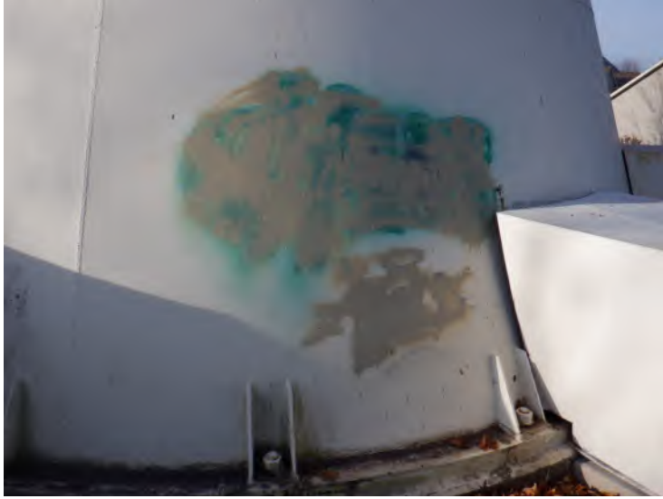
7) Coating failures on the basebell.
