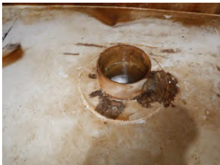
60) The fill/draw pipe is in good condition. There is not a deflector plate or bar over the top of the pipe.
