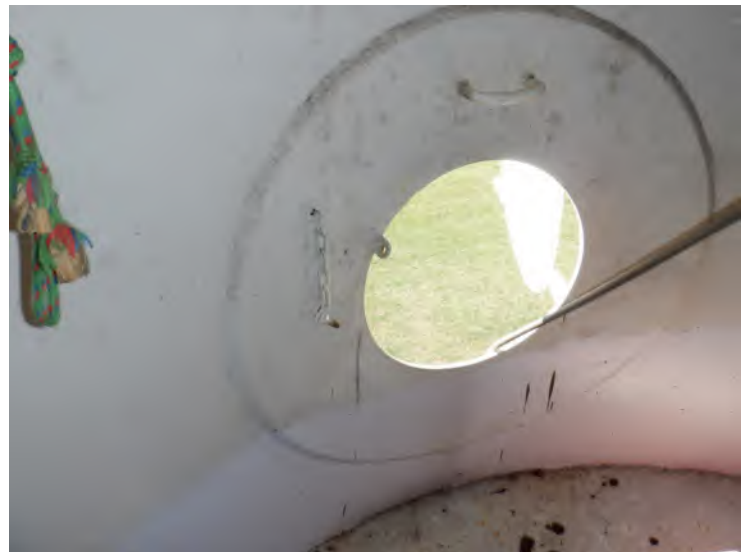
41) There is a handhold above the painter's hatch at the top of the riser.
