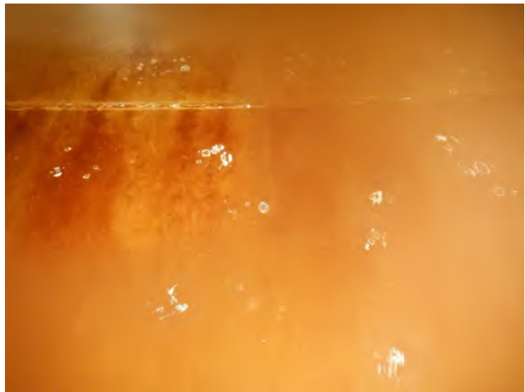
50) There are blisters in the sidewall coating on the lower sidewall panels.
