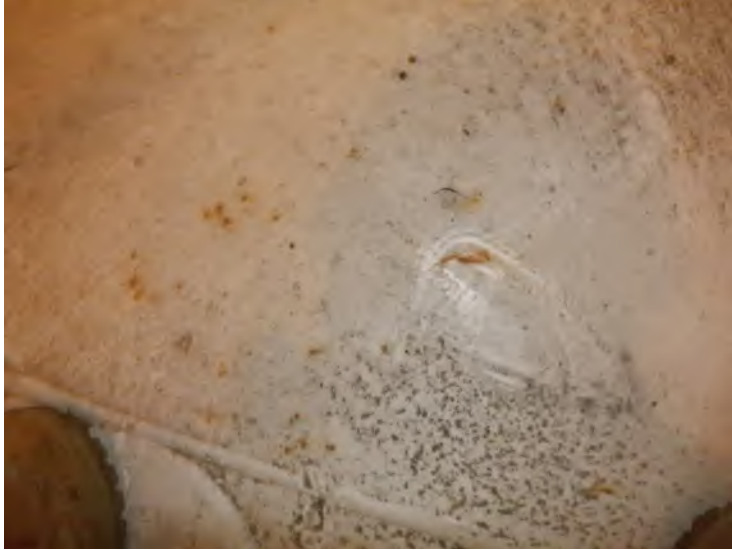
31) Minor coating failures on the condensate platform.
