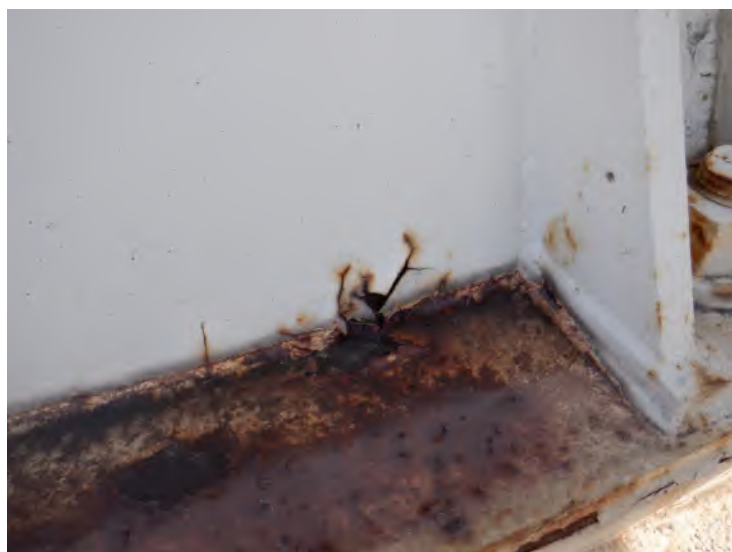
6) Coating failures on the baseplate.
