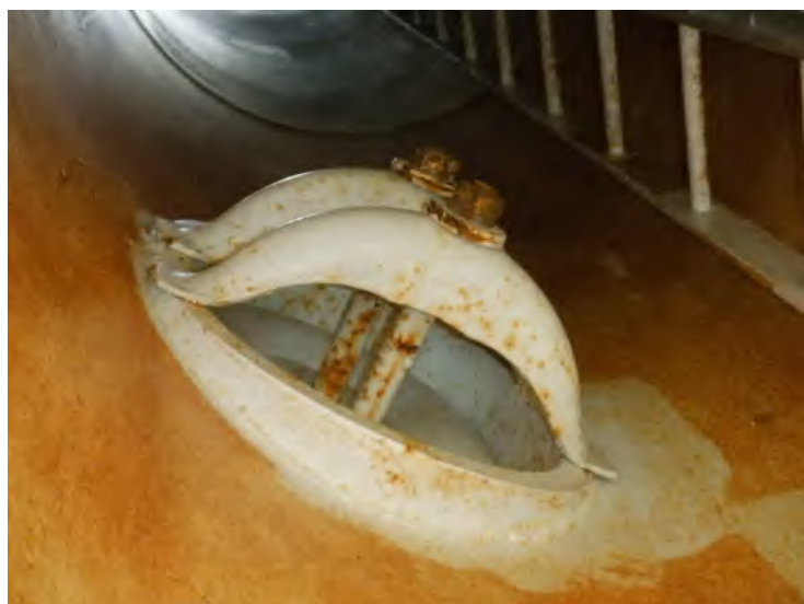
48) Coating failures on the wet interior manway.
