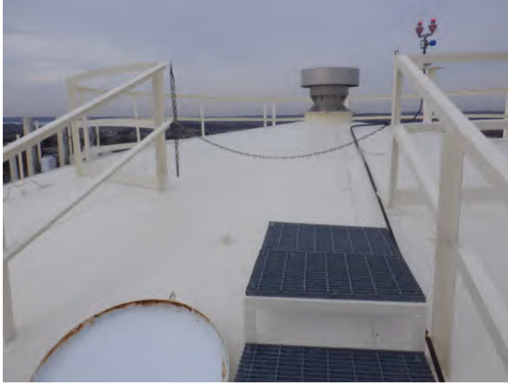
25) There are safety chains at the opening to the center handrail.
