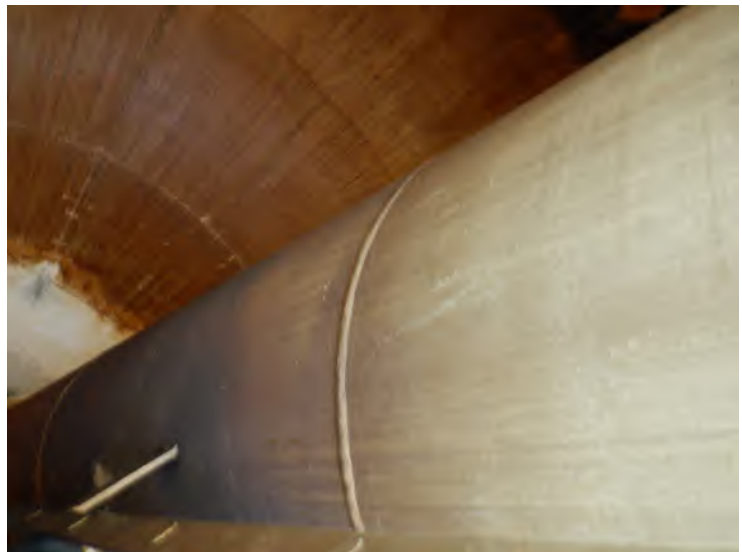
56) There are no coating failures on the access tube in the wet interior.
