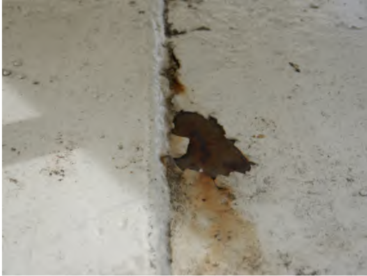
22) Spot coating failures on the roof.
