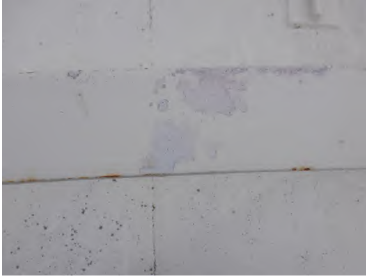
28) There is delamination along the handrail.
