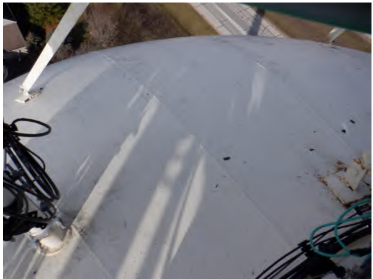
20) Coating failures on the roof.
