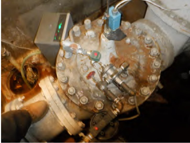
67) Minor coating failures on the pit piping.
