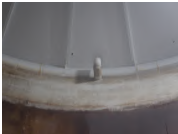
45) The overflow elbow is in good condition.
