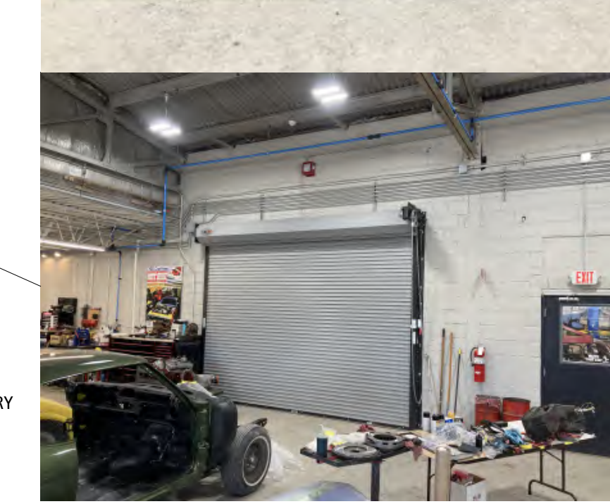
18 PHOTO OF 3-HR FIRE RATED O.H. DOOR 3" = 1'-0"
